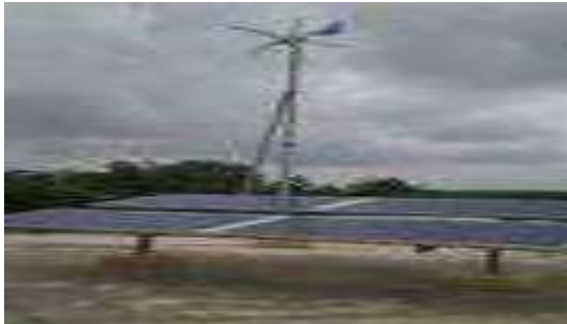
Fig (4) Wind Power Plant
