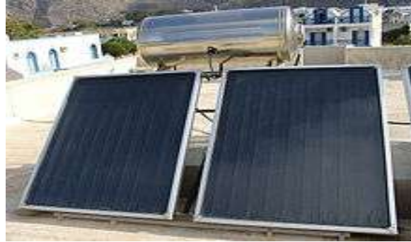
Fig2. Flat plate thermal system for water heating deployed on a flat roof.[6]
