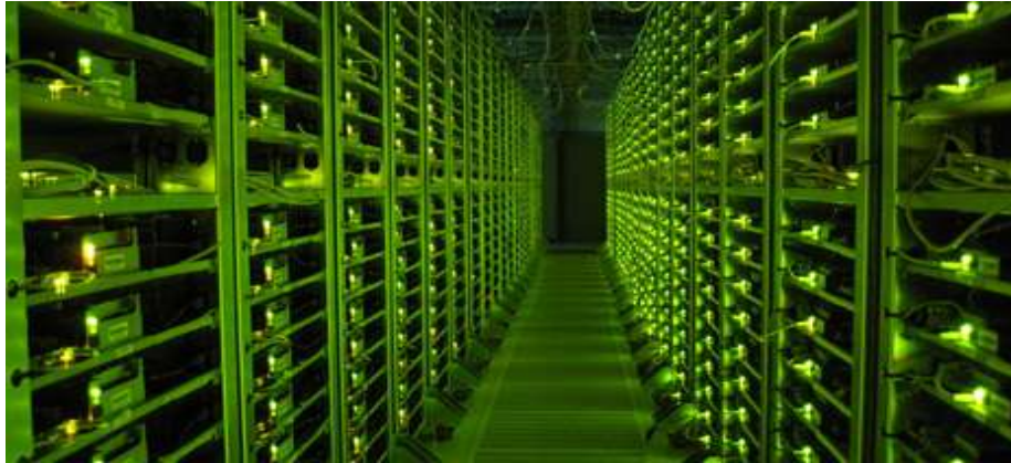
Figure 2: Green Data Center [16]
