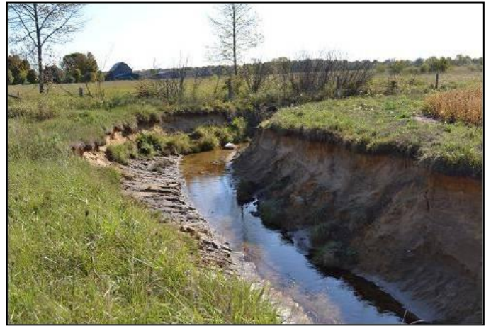
Fig - 4: Bank Erosion
