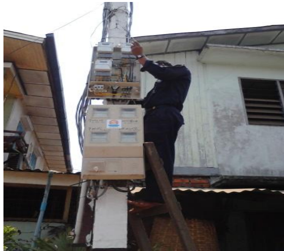
Fig 5 Installation of 1 Phase 2 Wire Offsite Meters Mounted on a Pole (with YESC Permission)
