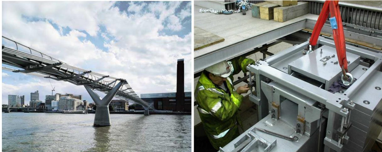
Fig. 4 Millennium Bridge in London and the Installation of TMDs
