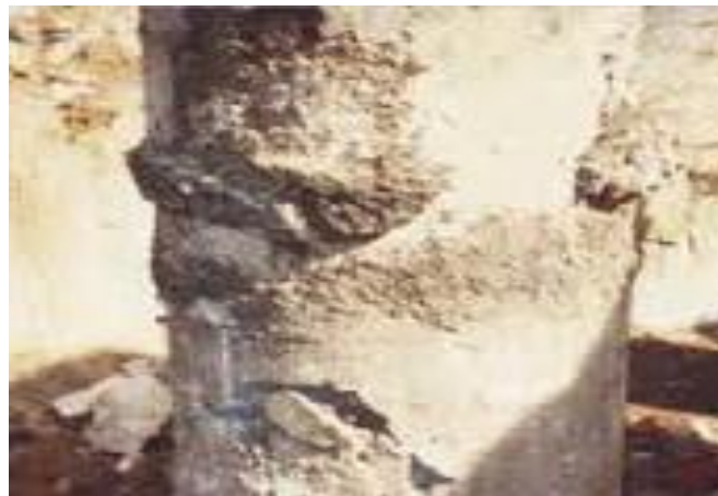
Fig. 11: View of defective pile after excavation.
