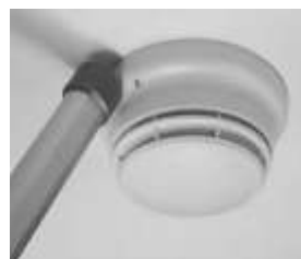
FIG 3. Simplex make 4098 smoke detectors
