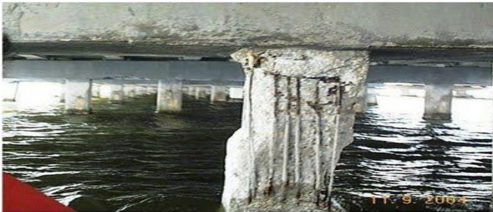
Fig.3.5 Impact damage that led to both cross-section loss and breakage of the spiral ties
