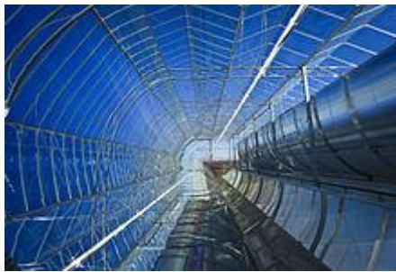
Inside an enclosed trough system
