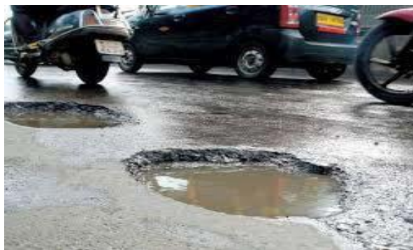
Fig. 1. Condition of roads with potholes.
