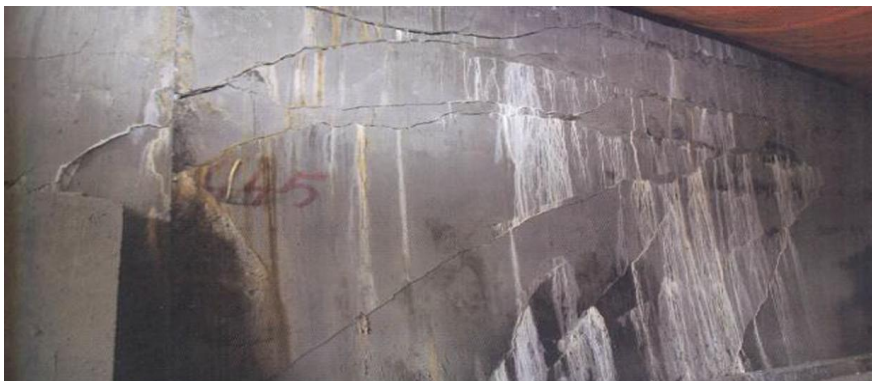
Fig. 4 Inclined cracking at the sidewall with water leakage and spalling.
