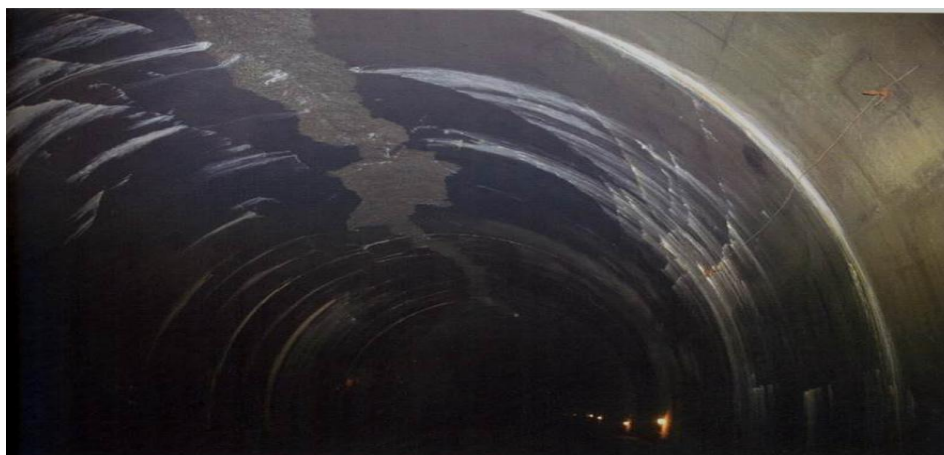
Fig. 2. Spalling cracking of the inside the tunnel.
