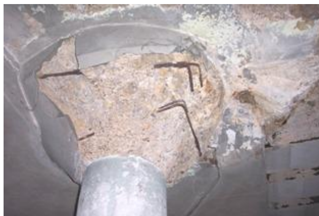
Fig. 5. Signs of deterioration of concrete
