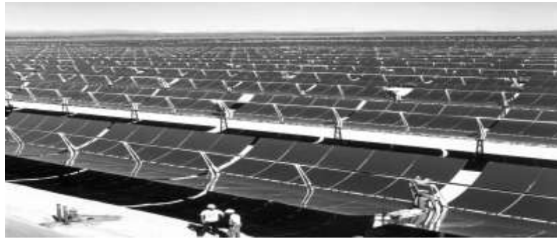
Fig-7 Solar Panels (Photovoltaic)
