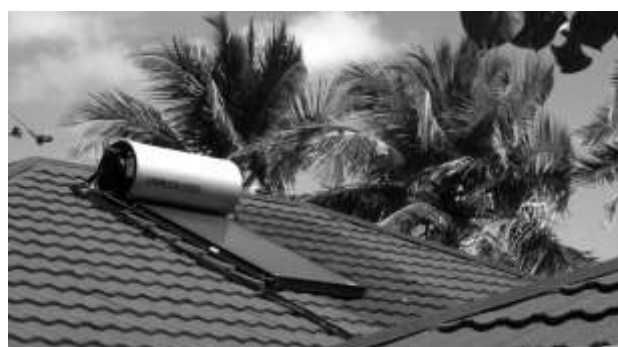
Fig-5 Solar Water Heater
